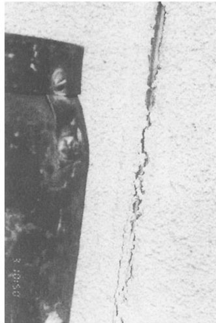
Figure 6 - Coating and sealant failure allows water to enter skin barrier systems.
