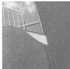
Broken granite cladding panel.
