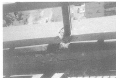
Figure 10 - Strong shadows cast by a railing obscures observation of the cracked concrete curb.
