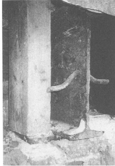
Figure 2 - This corroding steel beam was found when the masonry in Figure 1 was removed.
