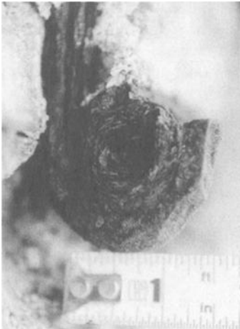
Figure 5 - This photo was taken with magnifying filters. Note the multiple rust layers of the hanger support.
