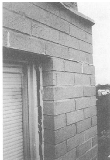
Figure 4 – Rust-jacking induced bulging at window corner.
