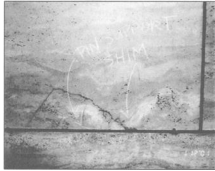
Figure 14 - Distress in stacked travertine panel at shim support
