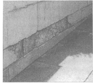
Exfoliation due to excessive water entry.
