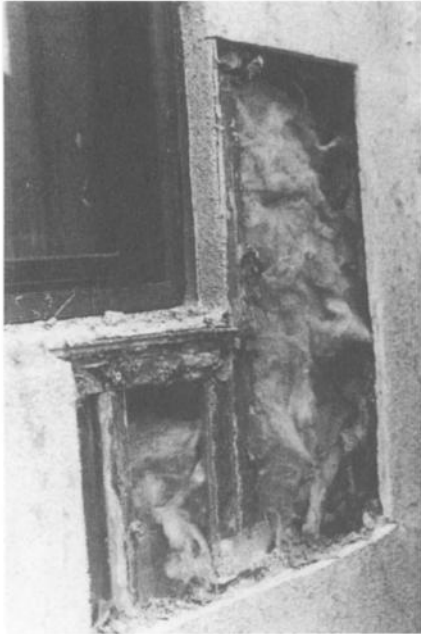
Figure 5 - Water leakage through this skin barrier stucco system has caused corrosion and other damage to interior wall components.
