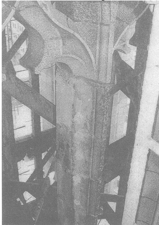
Figure 4 – Precast concrete used as a replacement material at the bell tower mullions
