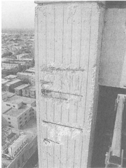
FIG. 2 - Example of concrete spalling distress in a building column.
