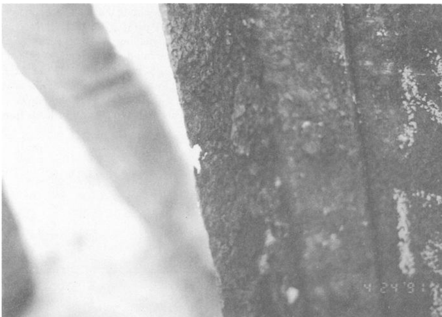
Figure 5 - Severe Corrosion of the Steel Column Flanges
