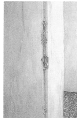
Failed sealants at cladding joint.
