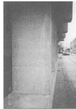
Unintentionally loaded limestone cladding.
