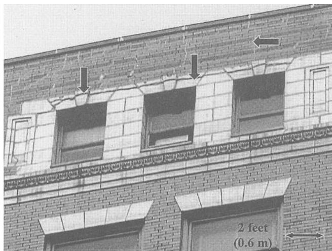
Figure 2 – Masonry Cracking Associated with Pack Rust
