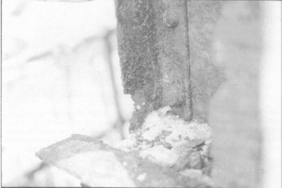
Figure 11 - Severe Column Flange Corrosion on Southwest Corner
