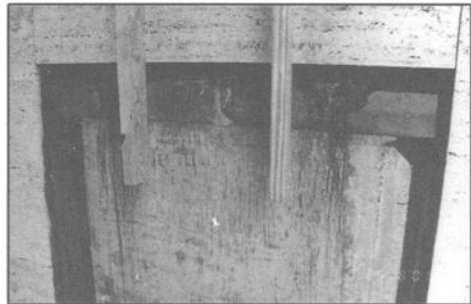
B. Corrosion of backup that resulted in stone panel displacement shown in Figure 3C
