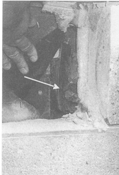
Figure 4 - Unsealed flashing at corner. Arrow indicates open end of metal flashing. Also note mortar blockage.
