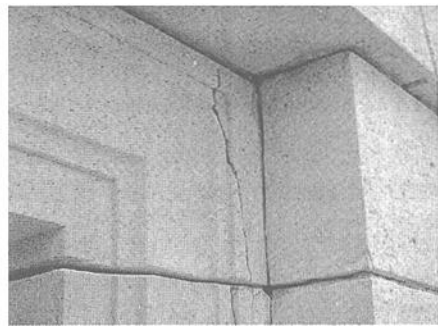
Figure 2 – Crack in granite window header about 500 mm (20 in.) long. Not visible from grade.
