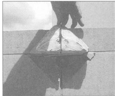
Figure 11 - Spalled limestone panel corners at ferrous washer
