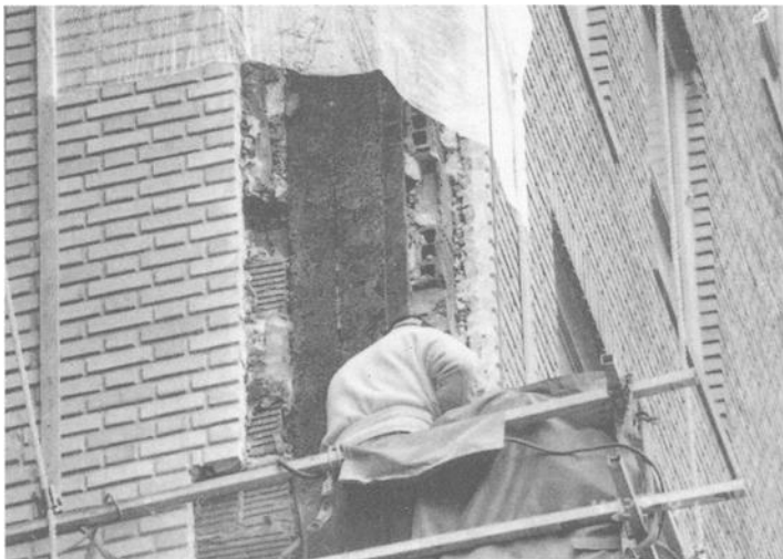
Figure 4 - Typical Corrosion of the Steel Columns at the Building Corners
