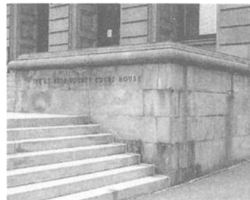
Soiling and staining of stone features.
