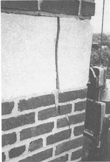
Figure 1 - Cracked and displaced masonry
